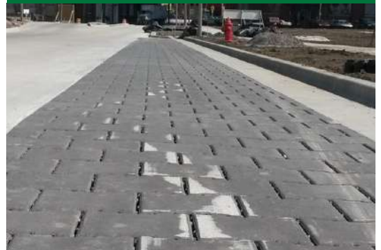
Can Plow and Seal To Prevent Salt Damage
