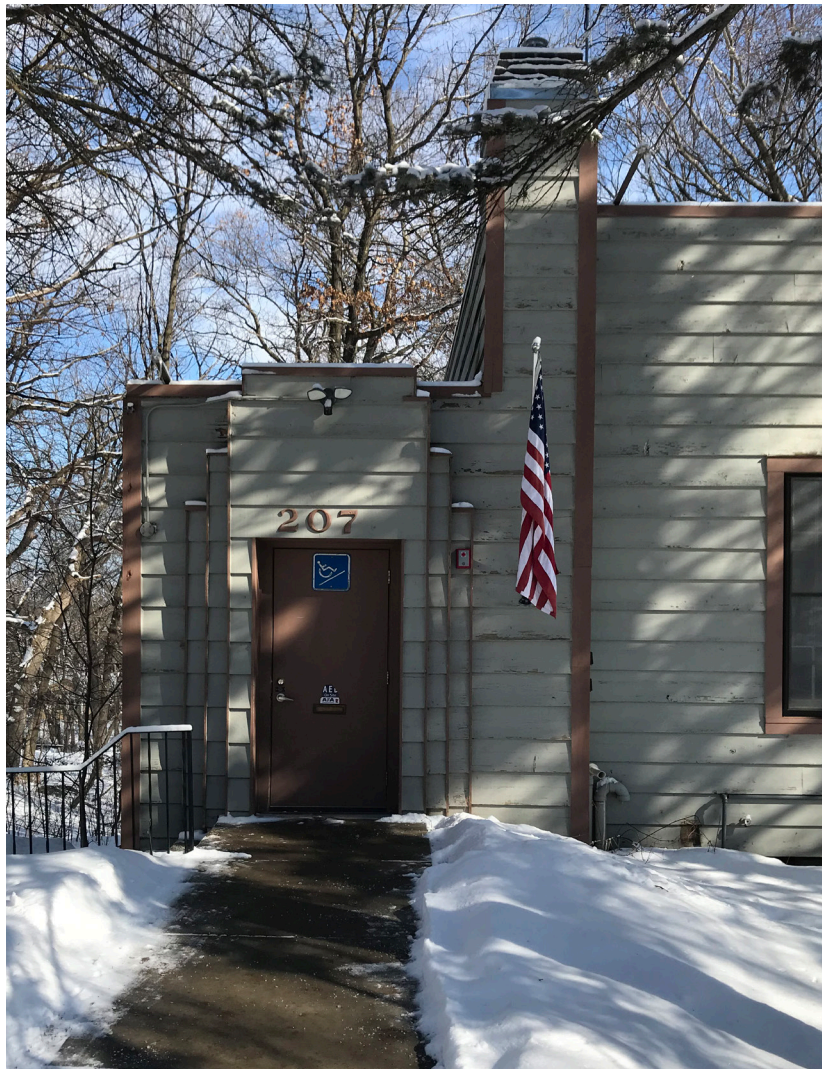
Main entry and chimney. Note stepped Moderne massing. Horizontal siding was added in the 1970s directly over top of the original vertical log siding.
