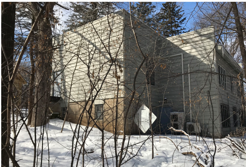
Southeast and Northeast elevations. Two level 1980s addition can be seen here at the rear (northeast) side of the building. Note Original tuckunder storage area adjacent to the 1980s addition.
