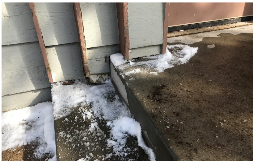
Detail view of stepped Moderne massing at main entry on southwest facing elevation. Note the presence of original half-round log siding revealed beneath the 1970s cedar cladding.
