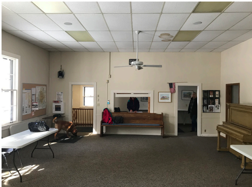
Main assembly room looking back toward entry foyer. note water staining on ACT ceiling, indicating roof issues.
