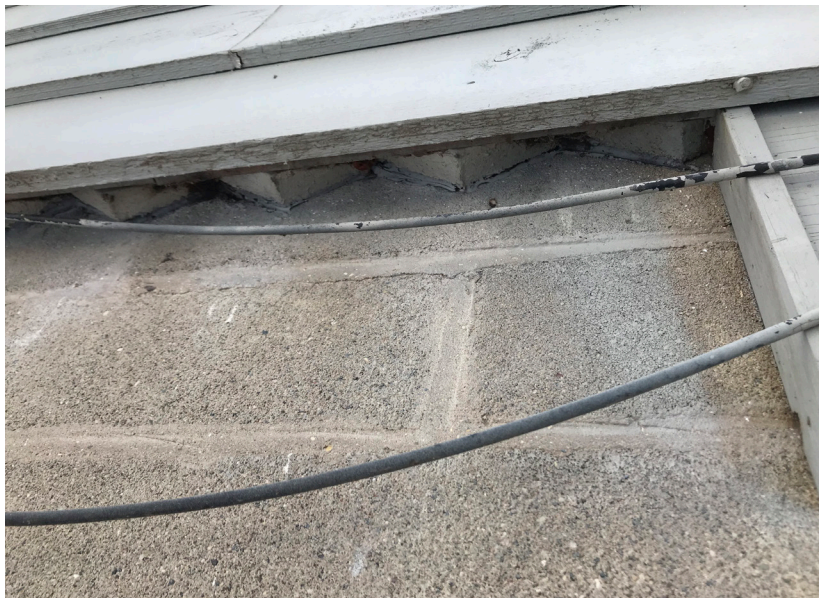
Additional evidence of original half-round log siding on the north elevation. This condition was observed around the entirety of the perimeter of the original building.
