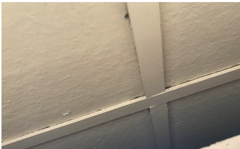
View of what may be the original ceiling above the current suspended ACT ceiling tiles.
