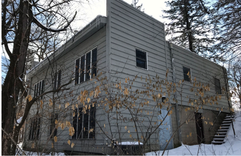
Two level walk-out addition constructed in the 1980s as seen from the northeast. The extent of the original building can be seen on the north elevation.
