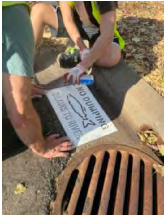
Figure 11 Storm Drain Stenciling
