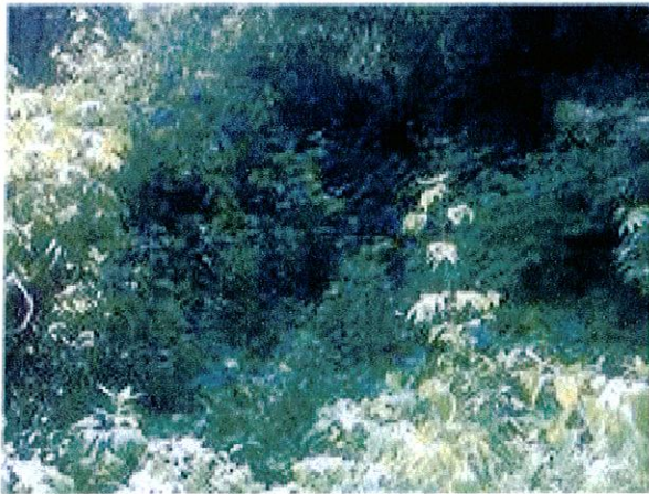
Example of overgrowth on the outlet
