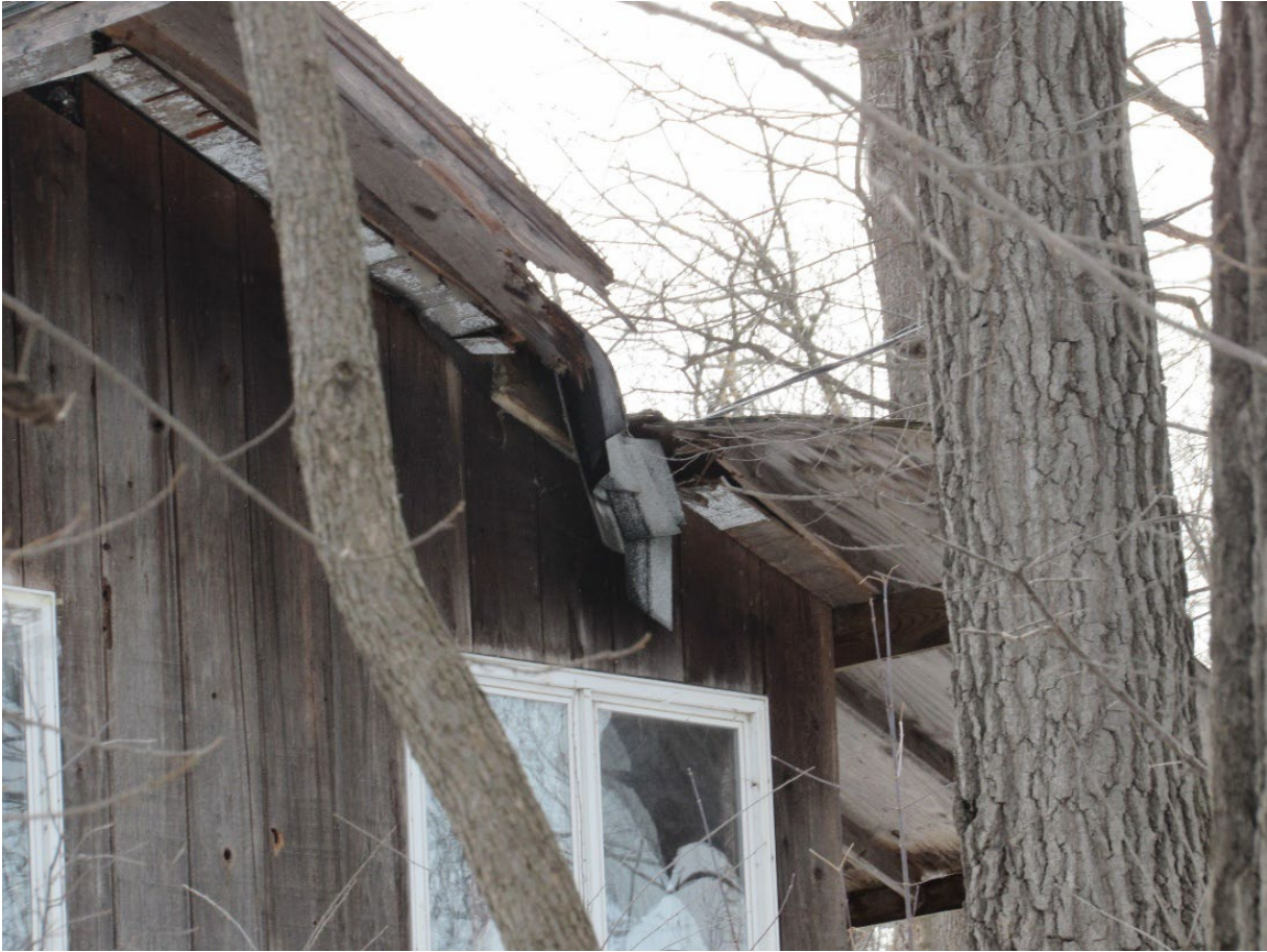
Damaged eaves, soffit and roof on north side of 310 (3/29/2024):
