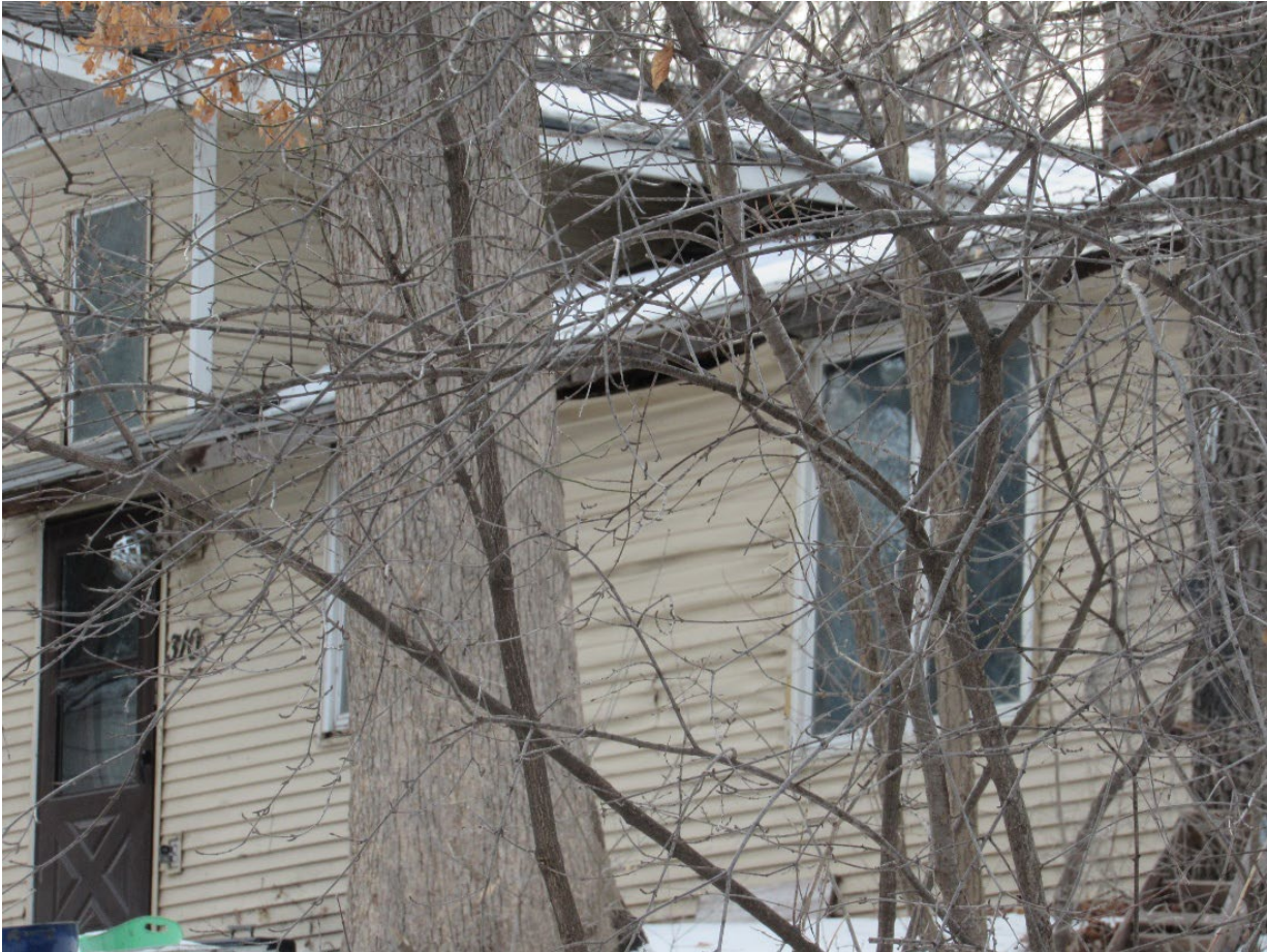
Damaged (wavy, likely from moisture) siding on east side of 310 (3/29/2024):
