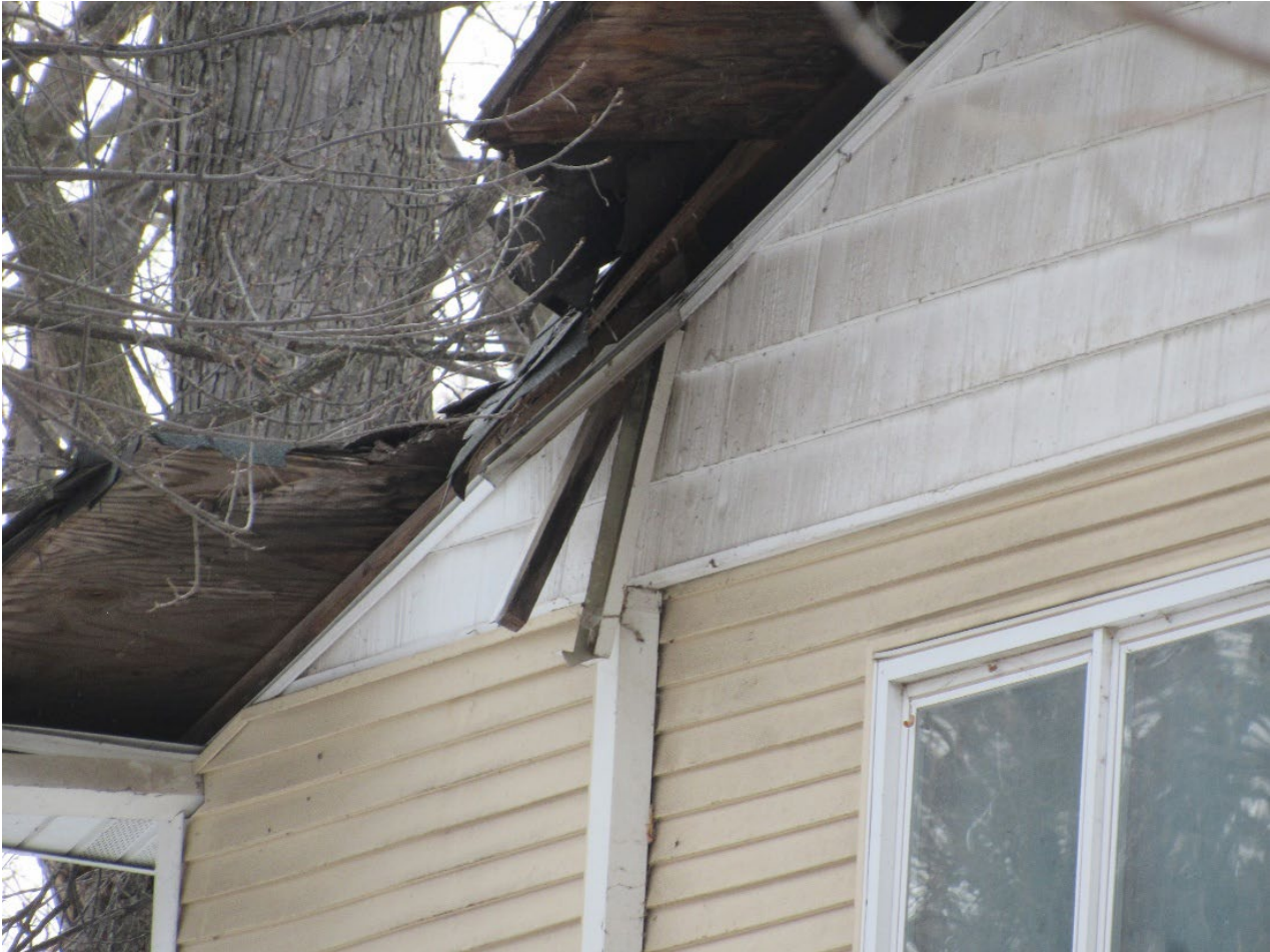
Damaged eaves, soffit and roof on east side of 310 (3/29/2024):
