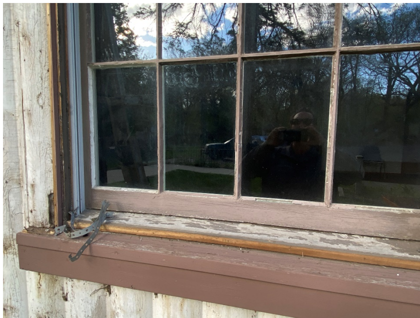
Figure 1 North window on west elevation showing vinyl jamb liner, decayed jams, and failed glazing and paint.
