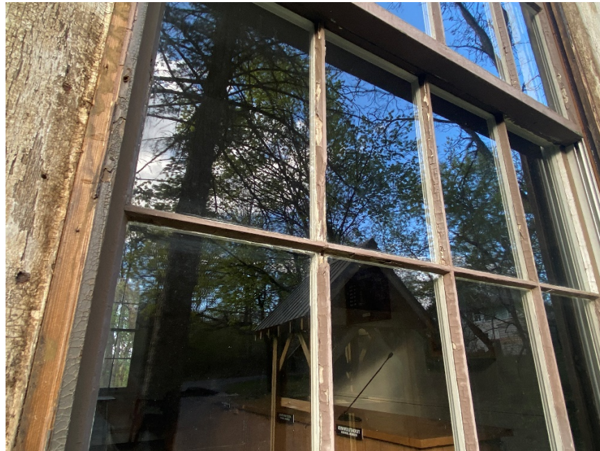
Figure 2 South window on west elevation showing damaged muntins, failure of glazing and paint, and decay of jambs.
