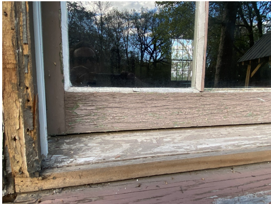
Figure 3 Middle window, west elevation showing paint failure and significant splitting and checking, paint failure and decay of frames and jambs.
