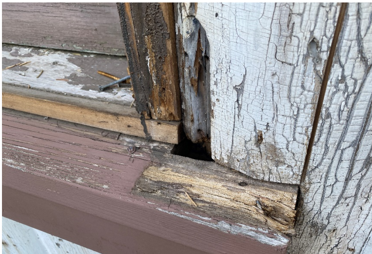
Figure 1 This photo shows the poorly fitted window sill and rot.
